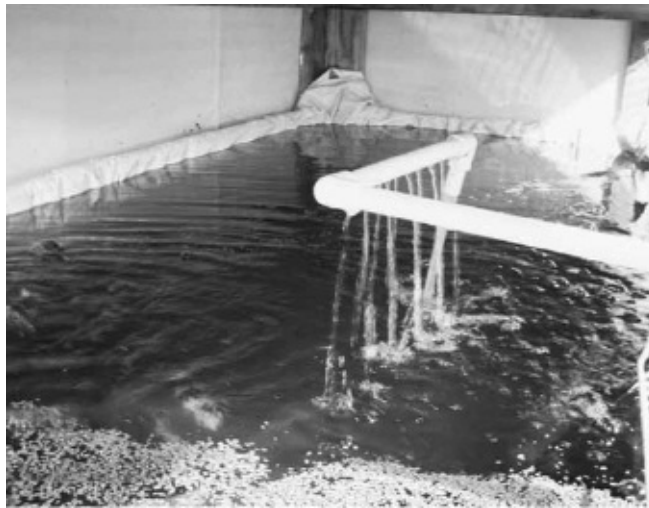
Aerating spray bar.
